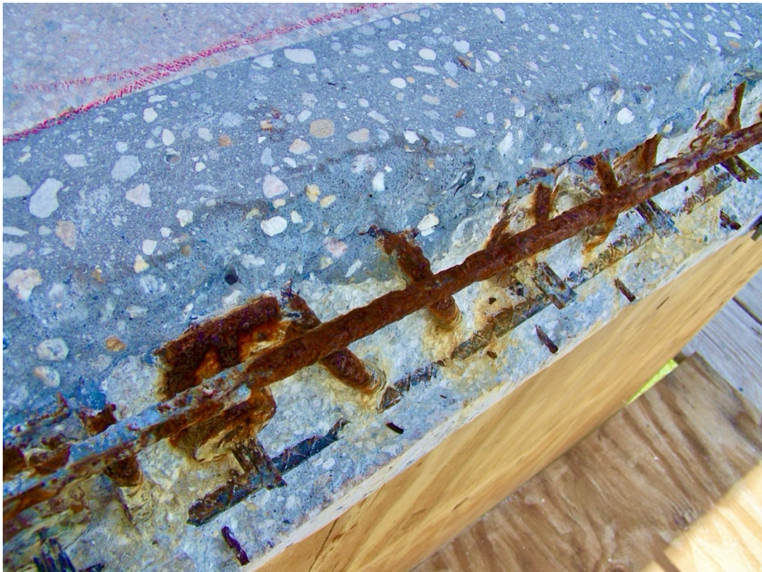
Photo: Old patching material is clearly visible, exposing advanced corrosion of embedded steel.
