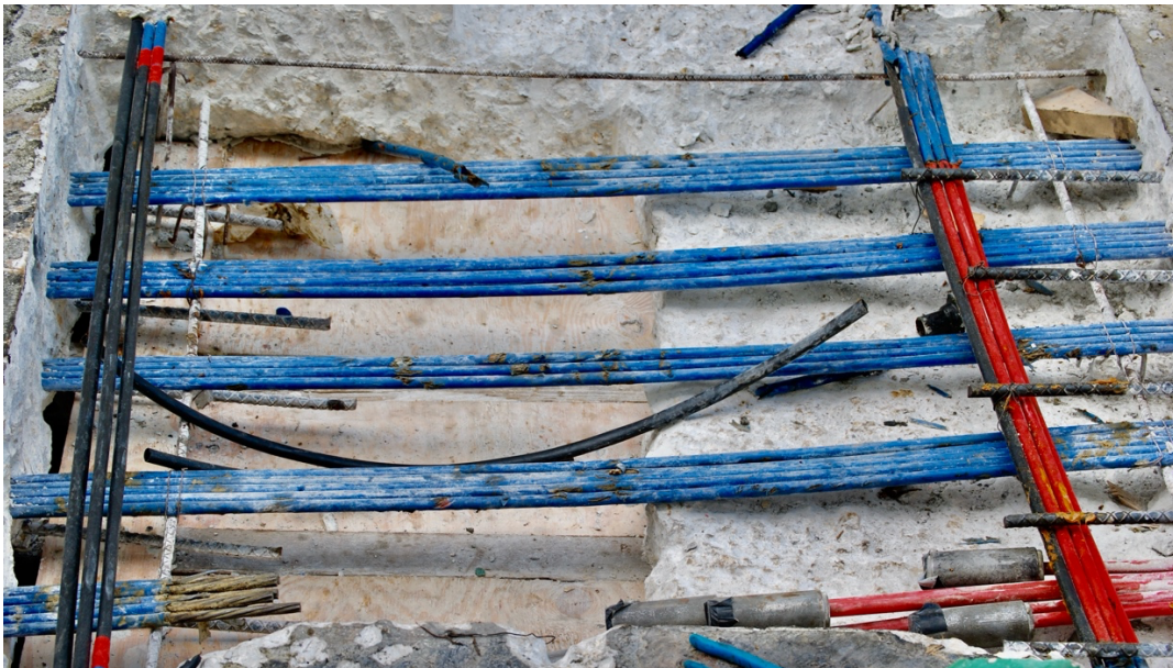
Photo: Groups of bundled tendons in a slab band line that is under repair.
