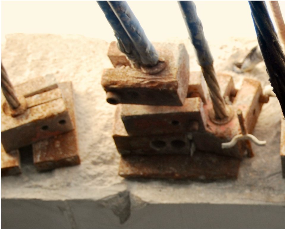
Photo: Bundled cables secured using single cable lock-off anchor that are stacked together.
